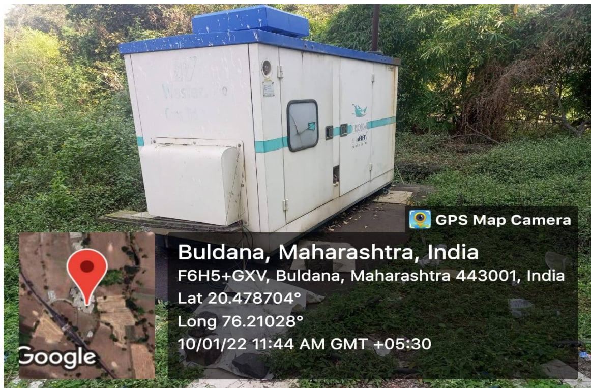
Diesel Generator Set
