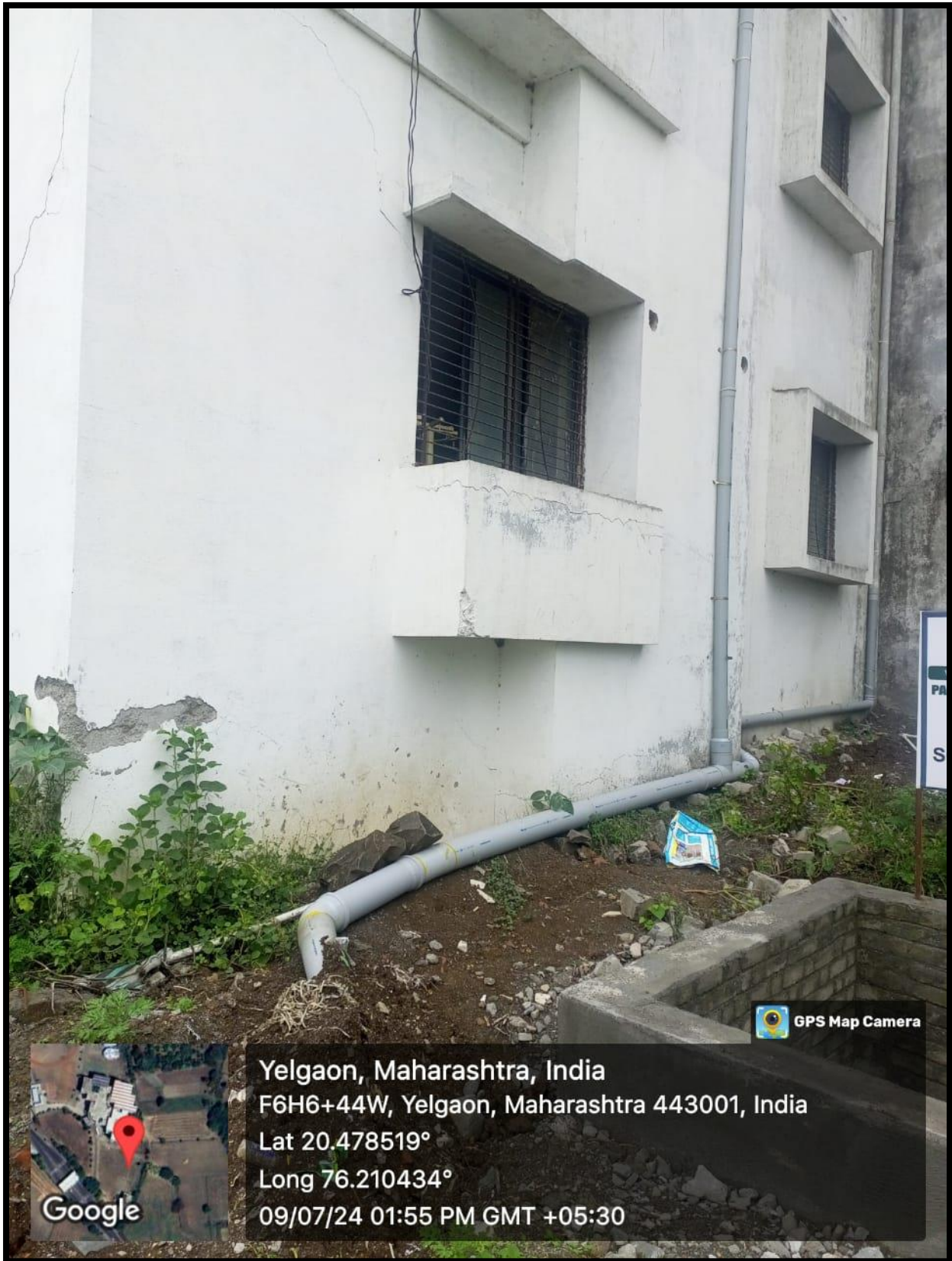
Rain Water harvesting Pipe arrangement
