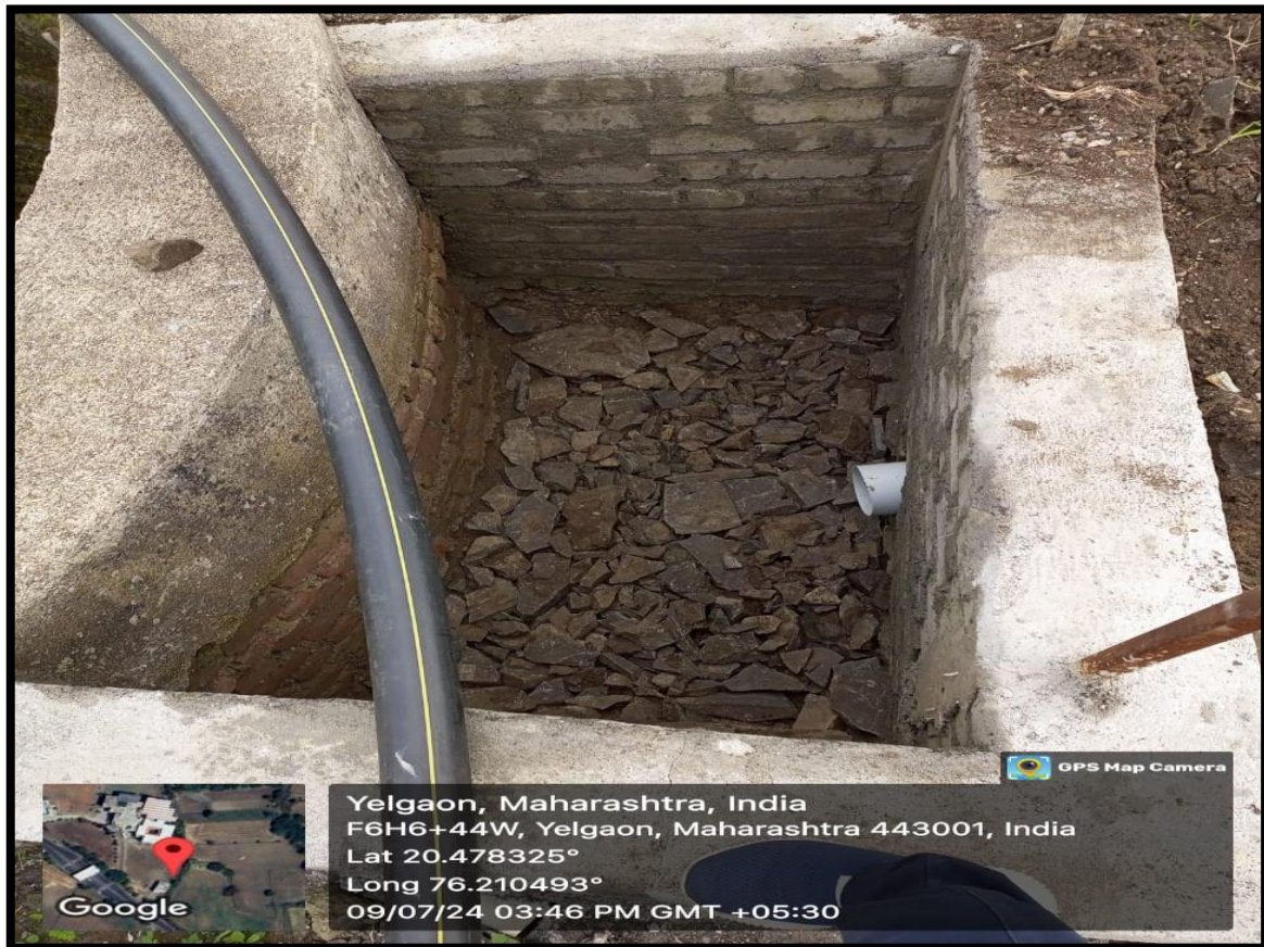
Rain Water Harvesting Pit
