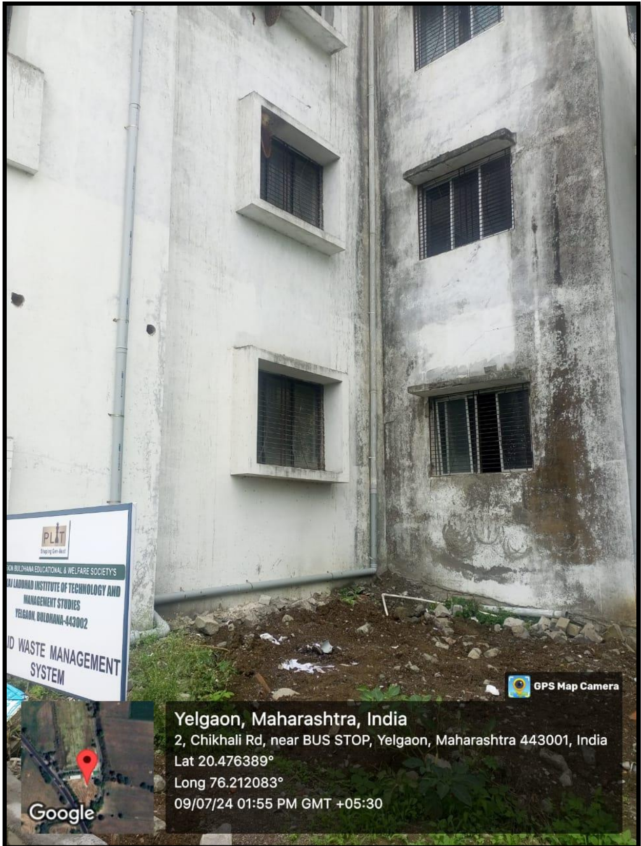
Rain Water harvesting Pipe arrangement
