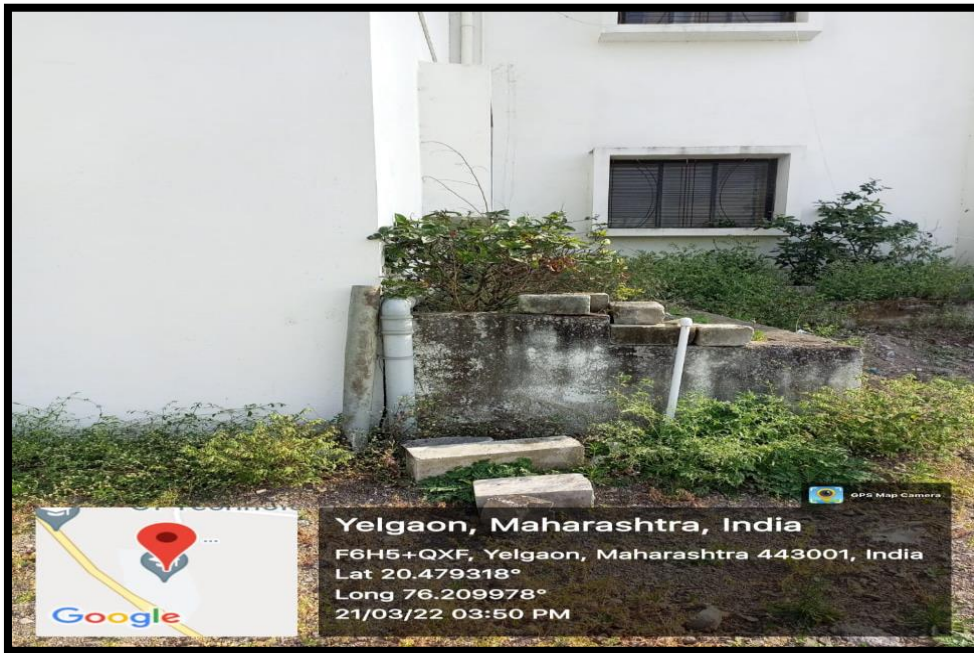
Rain Water harvesting Pipe arrangement
