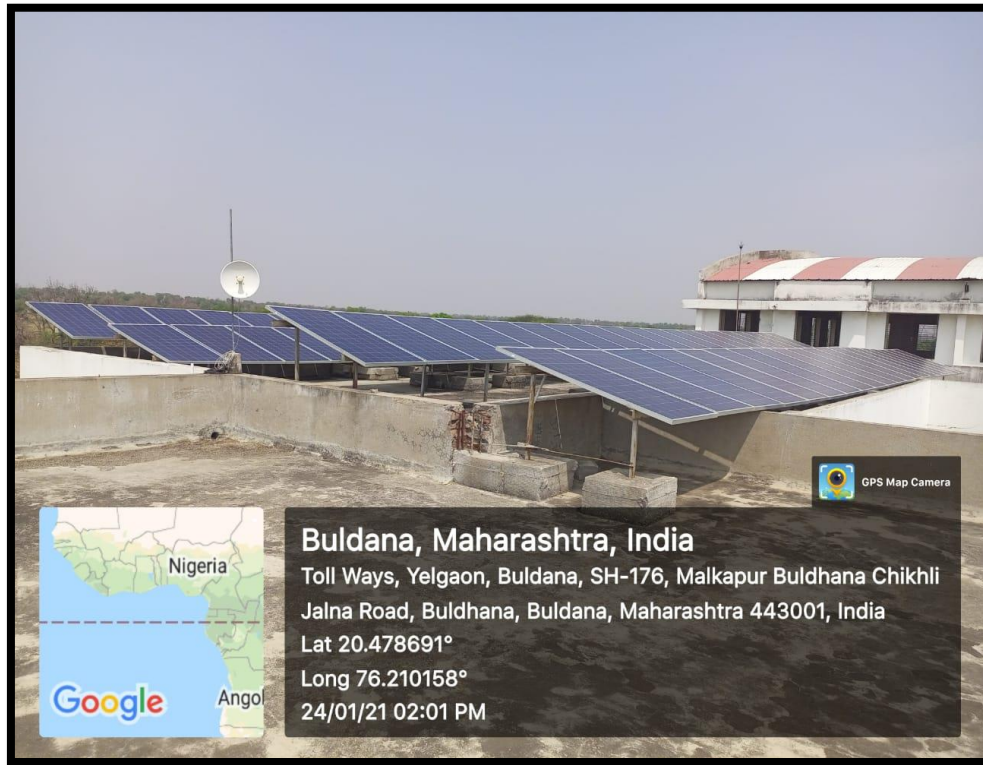
25 KW Solar Power Plant installed at Pankaj Laddhad Institute of Technology & Management Studies, Buldhana
