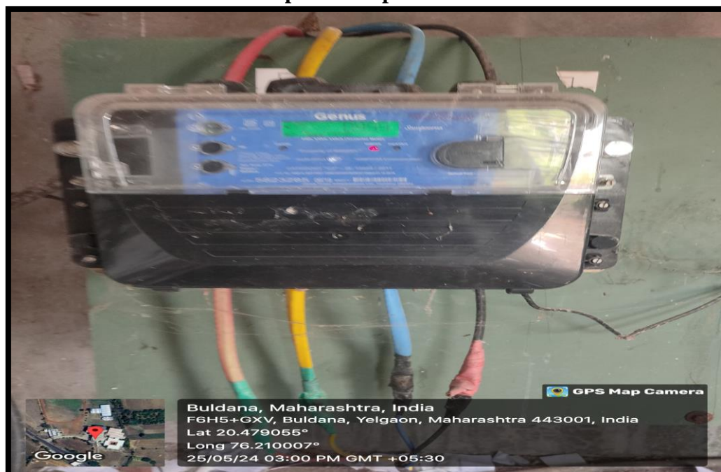
Solar Generation Meter
