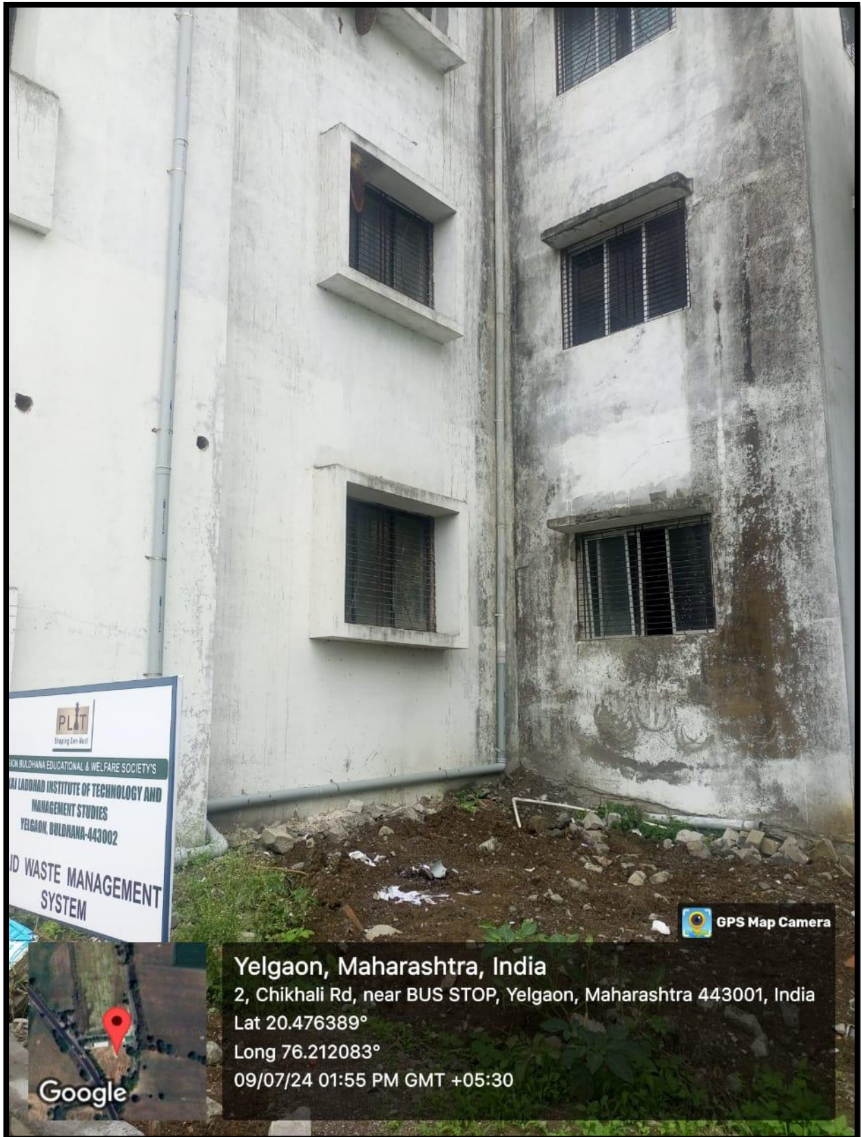
Rain Water harvesting Pipe arrangement
