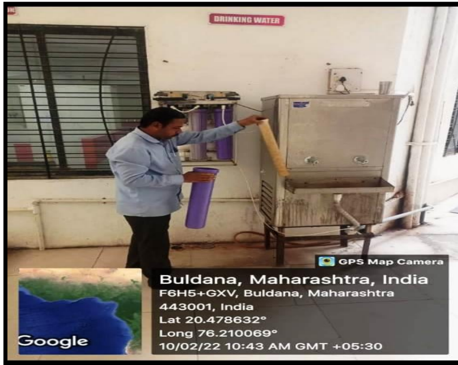
Water cooler maintenance carried out in every month
