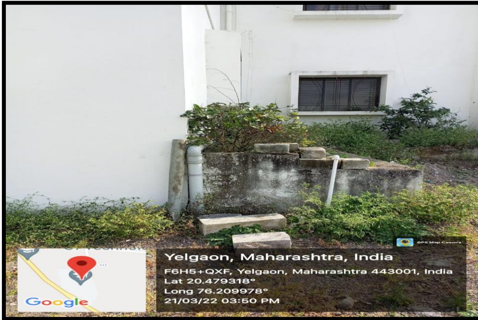
Rain Water harvesting Pipe arrangement
