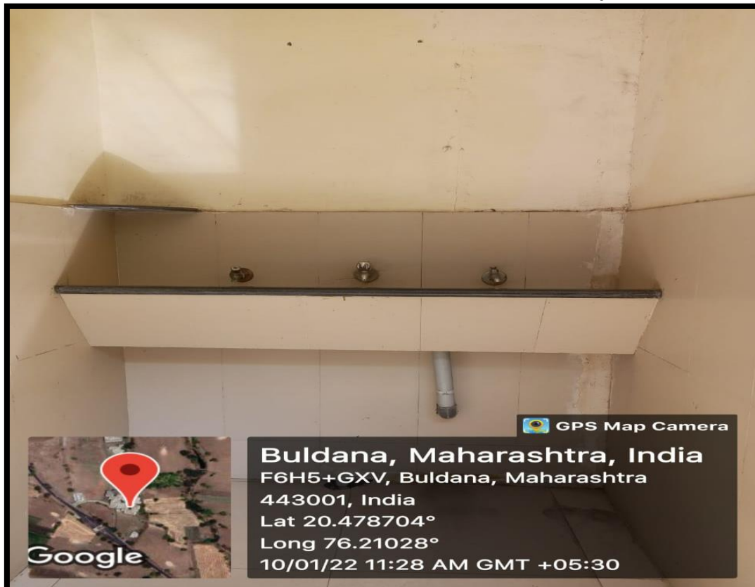
Wash basin facility available at various spot
