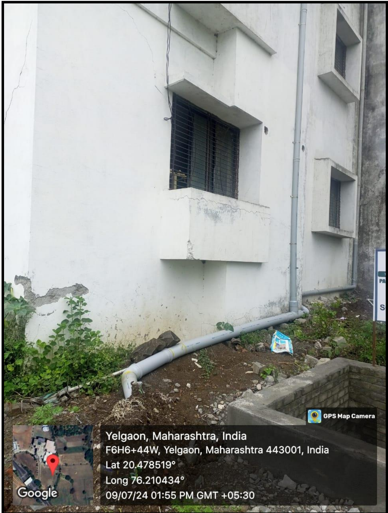
Rain Water harvesting Pipe arrangement
